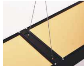
3.THE COMPLETION EFFECT OF THE SUSPENSION IS SHOWN IN THE FIGURE. 3. 吊線完成效果如圖示
