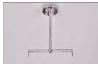
3. FIX THE BOOM TO THE CEILING WITH EXPANSION SCREW 3. 將吊桿用膨脹螺絲固定到天花上
